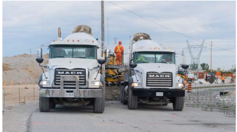
The Perimeter Access Road will provide access to local businesses surrounding the Canadian Point of Entry.
