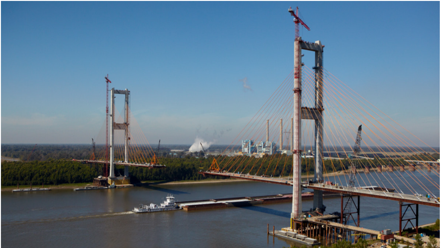
Example of stick build construction method: John James Audubon Bridge, Baton Rouge, Louisiana
