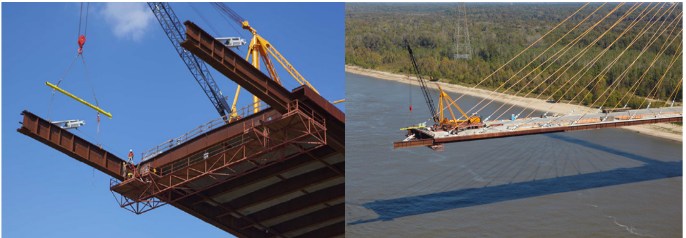
Example of stick build construction method: John James Audubon Bridge, Baton Rouge, Louisiana
