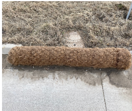
The coir log positioned in front of the drainage system
